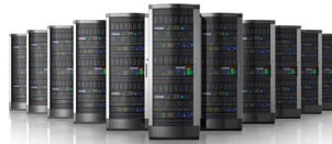
IoT and data center management
