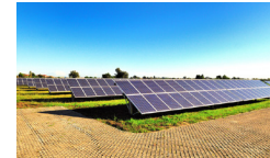
Solar and Inverters
